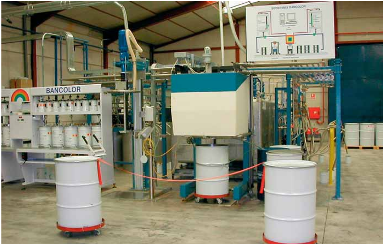
A semi-automated colour bank provides access to the global resources and support of the Becker Group for a marginal investment.
